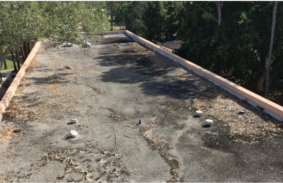
Lack of roof maintenance
