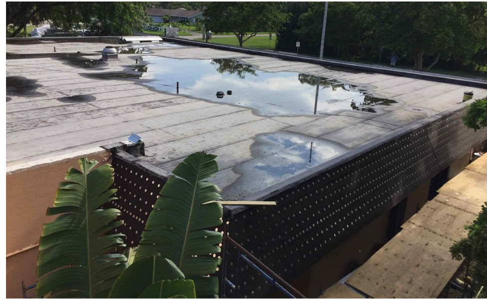
Lack of proper slope causing ponding of water on roof
